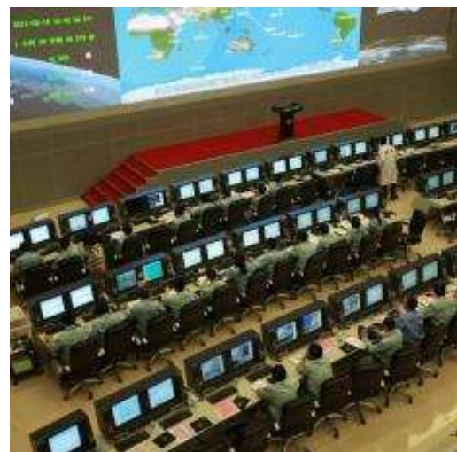
Fig.3 BACC Space Station Control Room [3]
